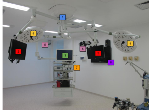
Figure 2. MIR elements in the room.
